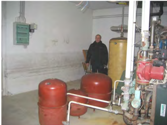
Picture of damage to equipment
